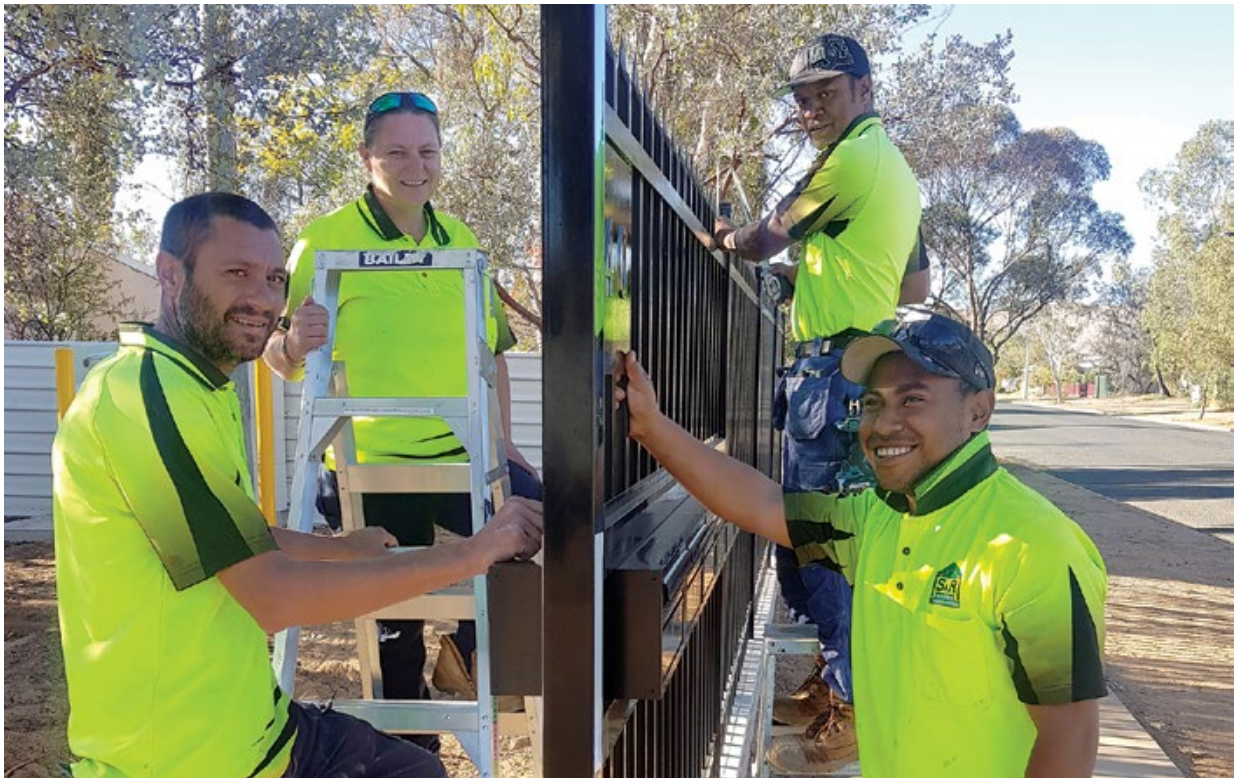
Work being carried out under the $100 million public housing stimulus program to improve security at 40 Albrecht Drive, Alice Springs
